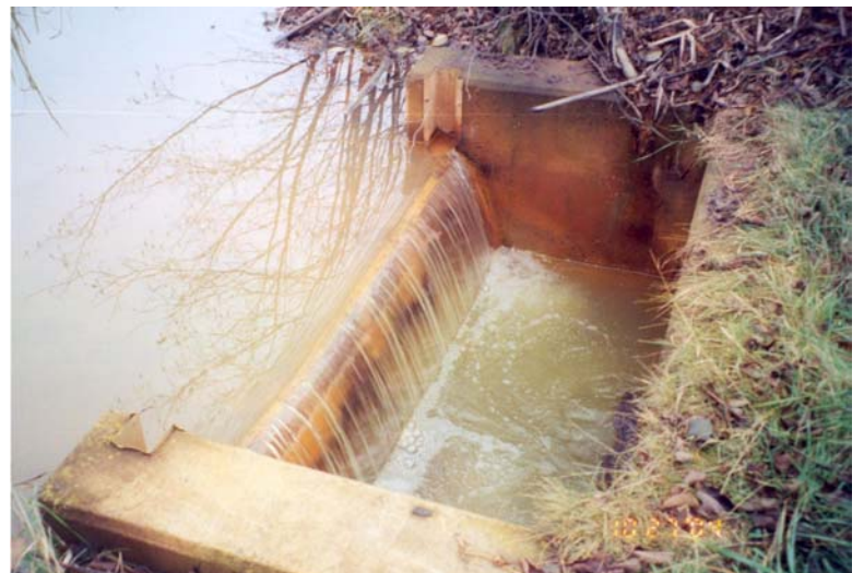
Photo 4 (bottom right). Dober Mine Synergetic Acid Water Treatment System outfall weir, 27 October 2004
